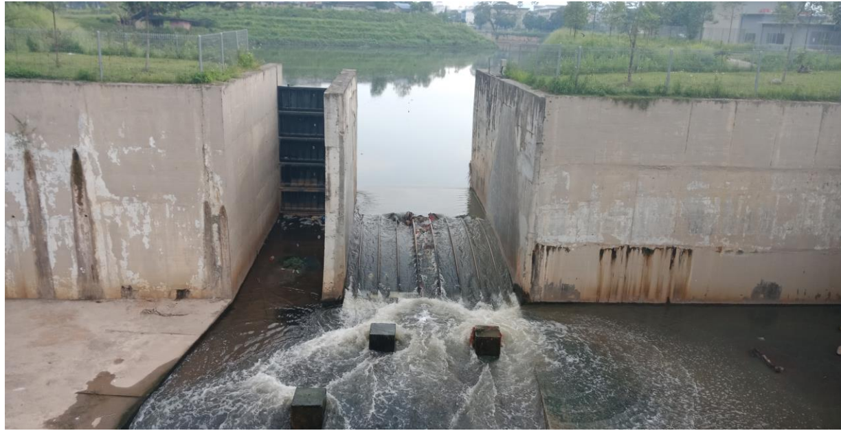
Water Control Structure (Obermeyer Gate)
