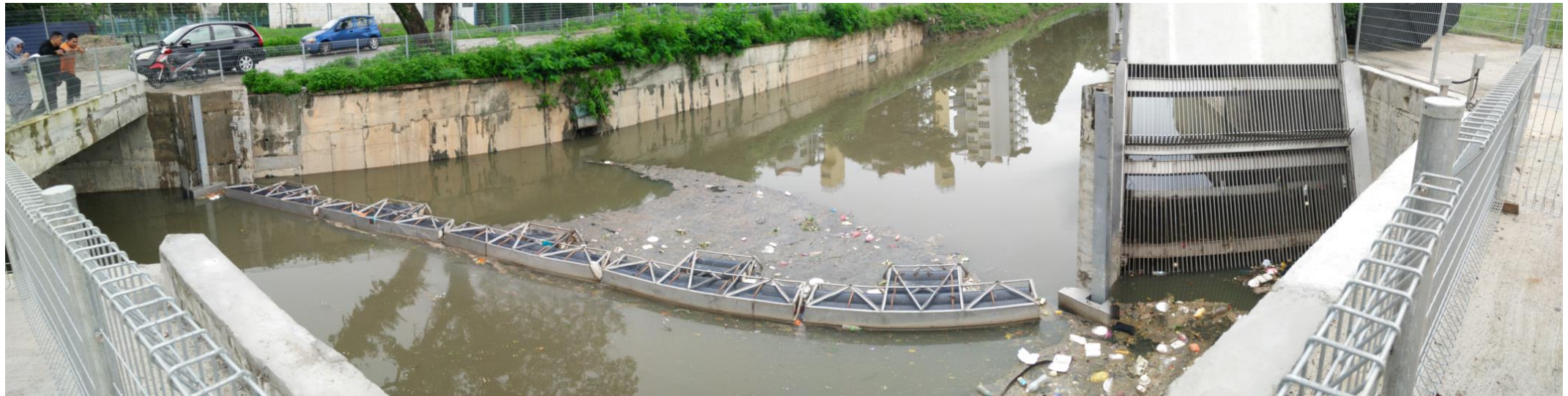
Mechanical Trash Rake and log boom
