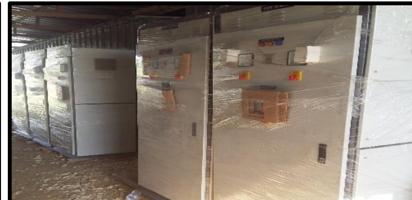
Control panel & cabling
